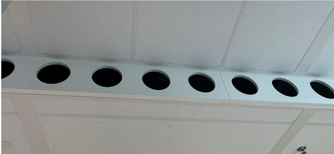
Figure 12: Exhaust air ducts of the exhaust & supply system to supply fresh air and for additional heating or cooling (own picture)
