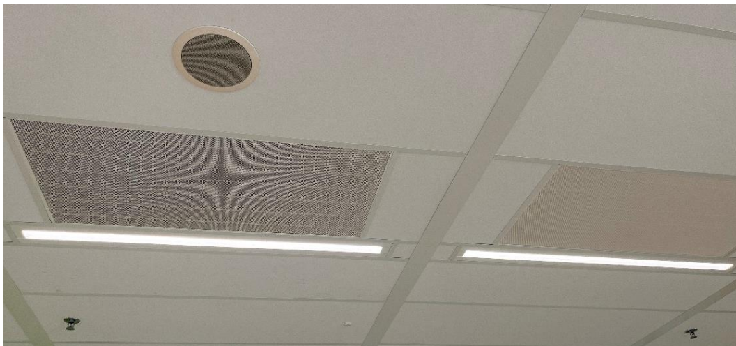
Figure 11: Active ceiling panels used for additional cooling in several rooms (own picture)
